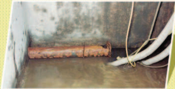
Dewatering by Pump with rusted Inlet
